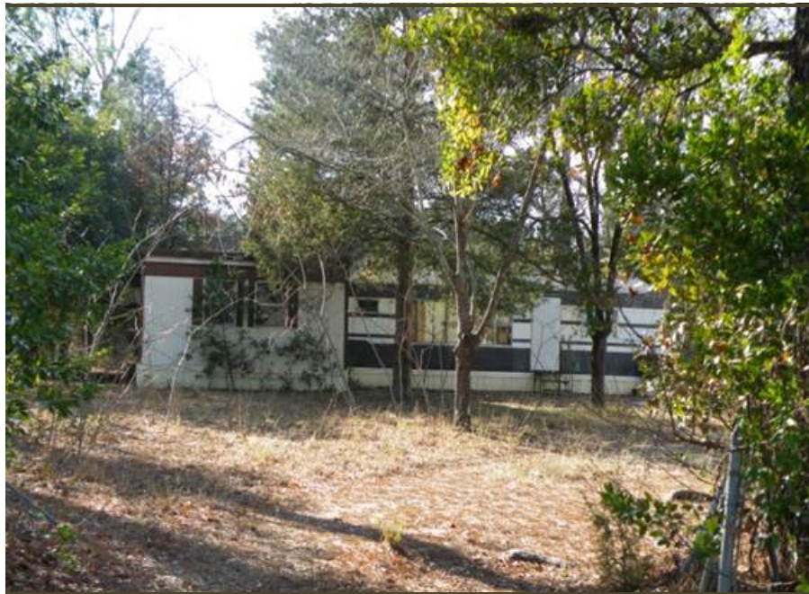
Vacant. Deteriorated. Concealed. A prime example of slum and blight in Grovetown. The aesthetics of many residential properties in the URP study area are serve to attract questionable activity.
